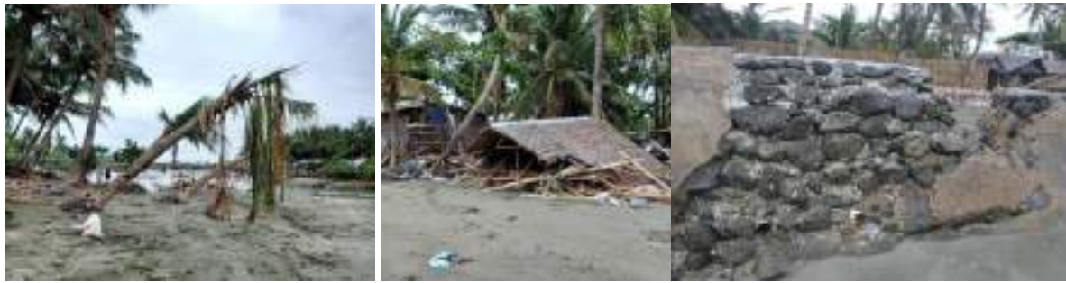
Figures 2. Barangay Agojo is highly exposed to strong winds, waves, and typhoons; The Agojo Seawall corroded within five (5) years of construction (Tagle, 2022)
